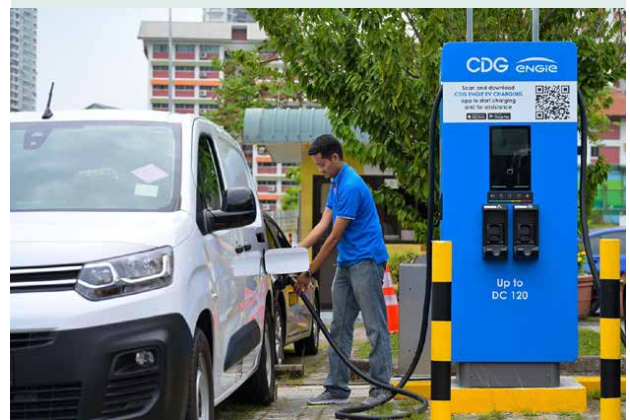
SETSCO collaborates with Starcharge in performing EV Charging Station (EVCS) inspection service to ensure public safety.
